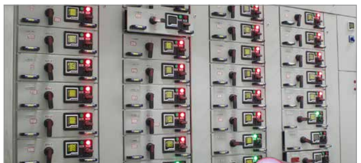
HV switching matrix
